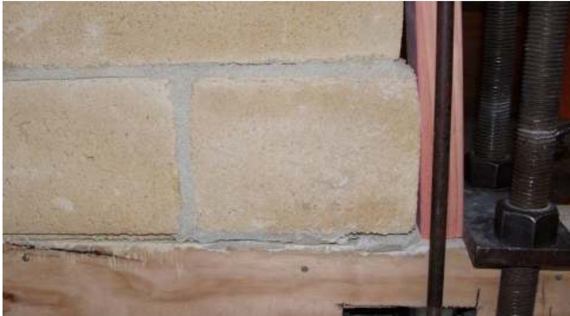
Photo 1: Shows cracking at 40mm top plate deflection, these cracks close up when top plate deflection returns to 0mm
