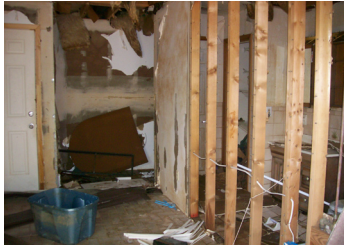
Internal Walls destroyed by Floods
