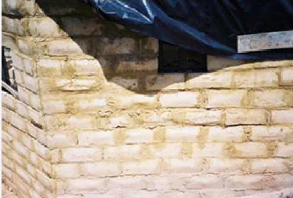
Sample of Incorrect laying of Timbercrete
