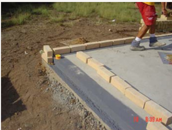
Term Seal and dampcourse coating being applied prior to laying Timbercrete bricks
