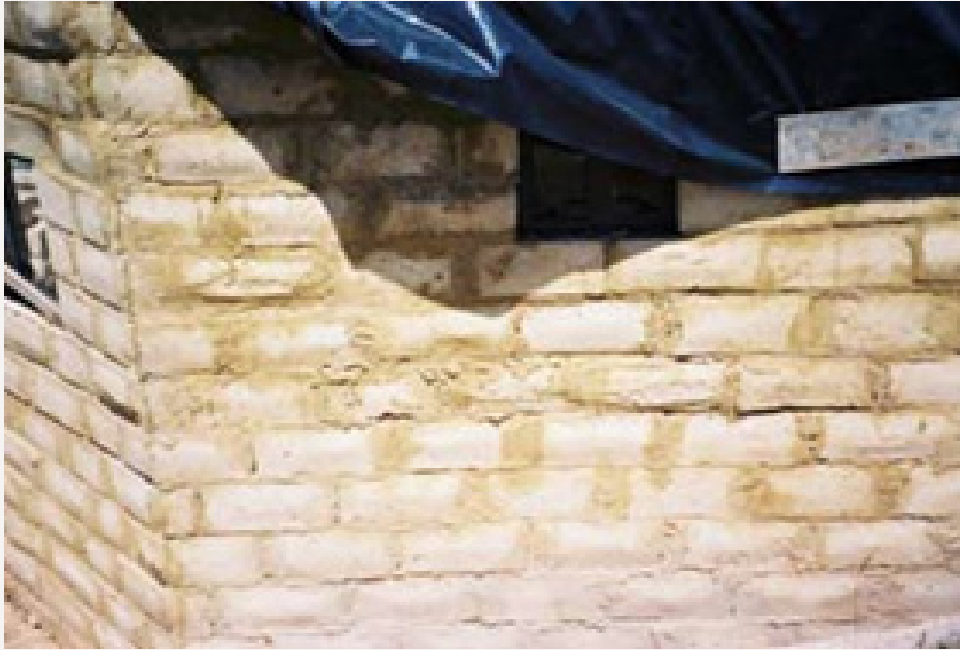
Sample of Incorrect laying of Timbercrete
